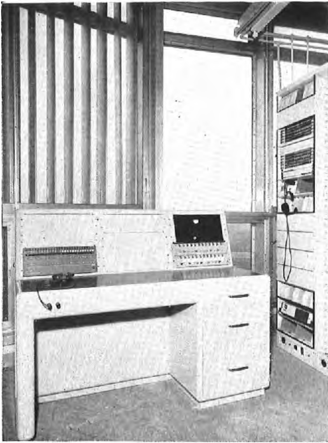
FIG. 19.—ALARM AND CONTROL EQUIPMENT. FLOOR B8
