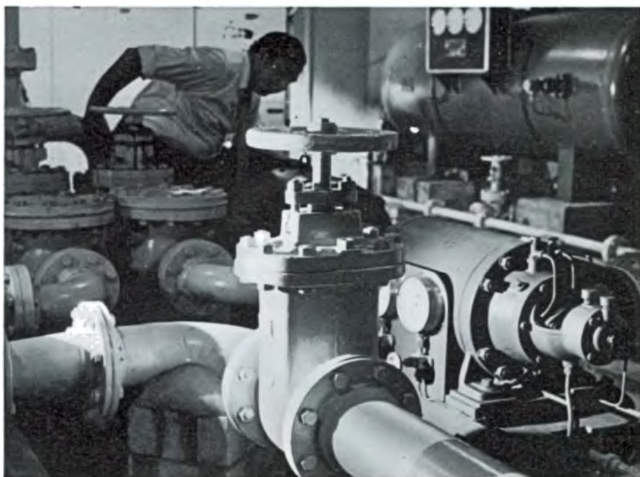
These fire booster pumps serving the Tower are installed in the new extension building.
