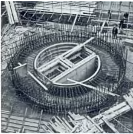
The foundations of the Tower were sunk 24 ft (7.3 metres) to rest on the hard blue London clay. A concrete raft, reinforced with pre-stressed post-tensioned cables, supports a concrete truncated pyramid. On this rests the 13,000 ton (13,208,000 kilogram) Tower.
