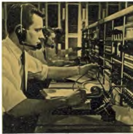
Trunk test desk: throughout the day and night technicians man testing positions from which a fault on any circuit can be rapidly identified and located.
