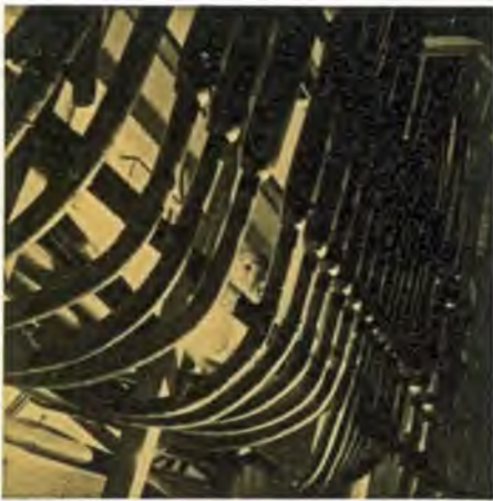
The main cable chamber in the basement of the building: underground cables rising up to the main distribution frame on the ground floor.
