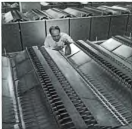
Inspecting the batteries: a maintenance man reads a hydrometer, an instrument for testing the specific gravity of the acid, in one of the very large cells. Batteries of these cells form an integral part of the power plant serving the telephone switching equipment.
