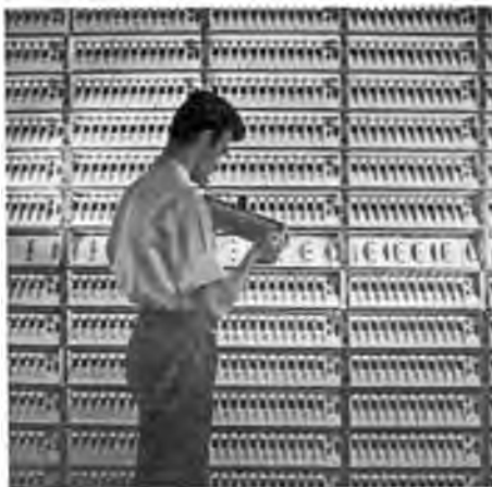
Inspection of a channel panel. One of these plug-in units is needed for each of the thousands of telephone trunk circuits brought into the Post Office Tower.
