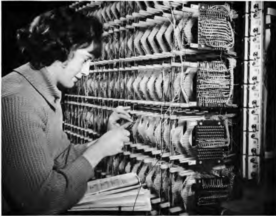
Fig. 3. Rack wiring of equipment for electronic telephone exchange Mark 2.
