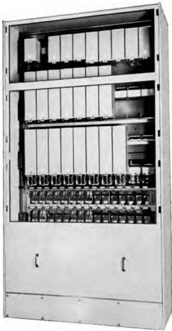
Fig. 2.— 10 + 99-Line P.A.B.X. in cabinet with some covers removed.
