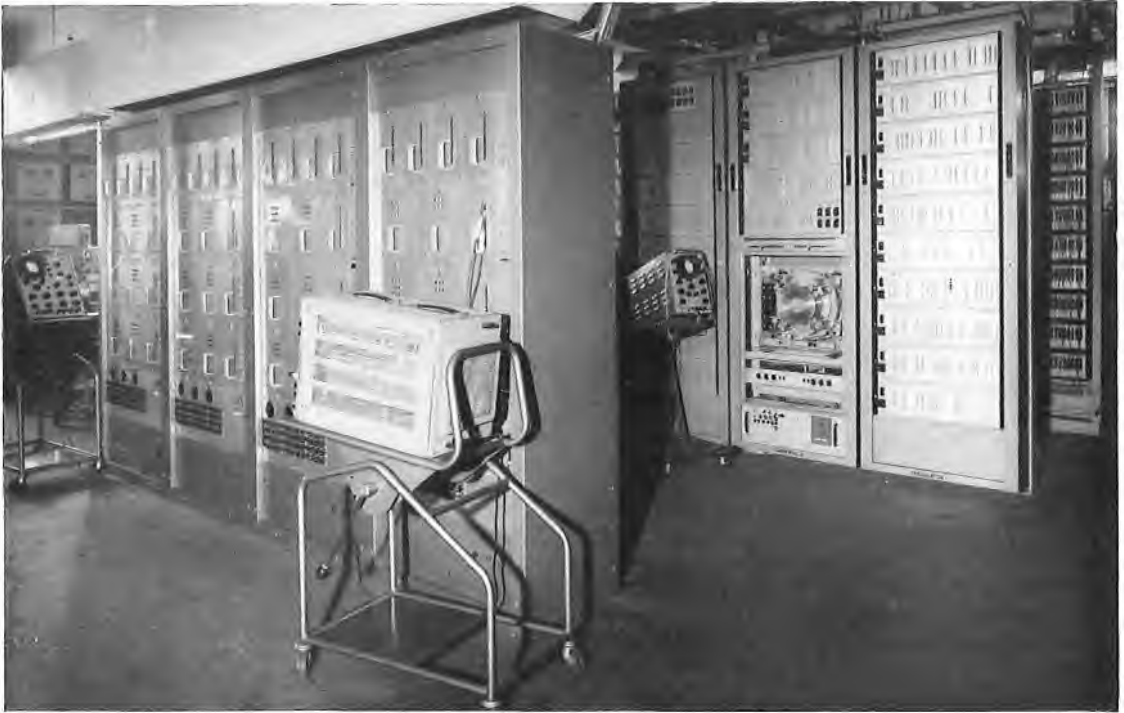
Fig. 4: General view of equipment racks
