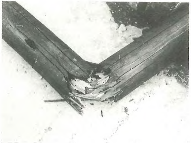
FIG. 7—Failure of brash pole
