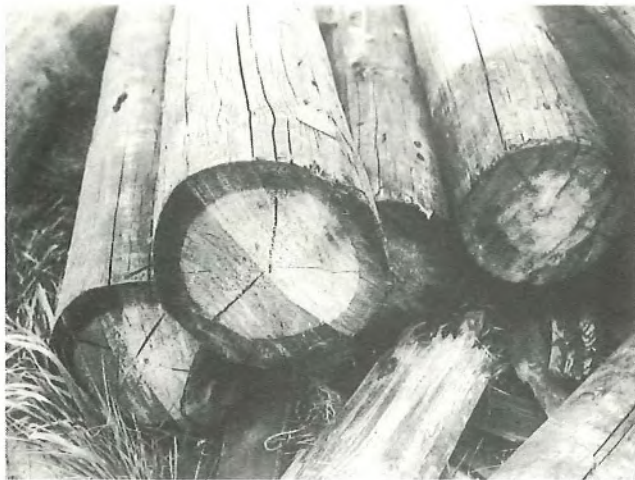
(a) Hardgrown timber with restricted creosote penetration
