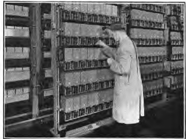
COMPLETED AUTOMATIC EXCHANGE IN SERVICE.
